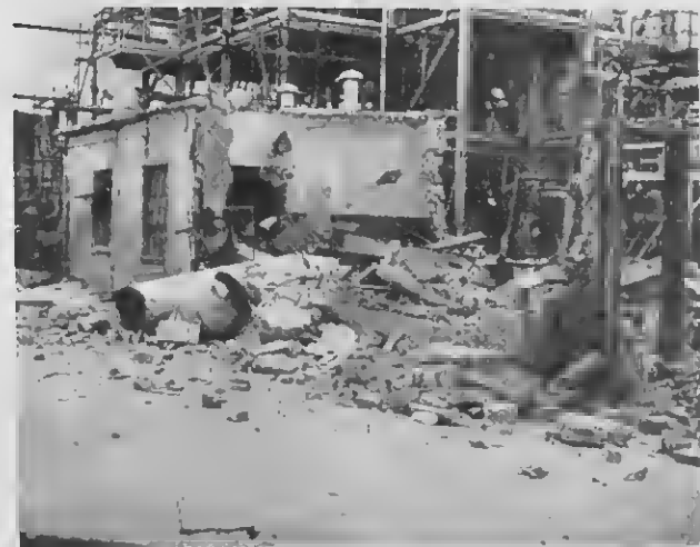
THE OLD control house was busted up in short order. These two views show the demise of the old low octane S & S control house.
